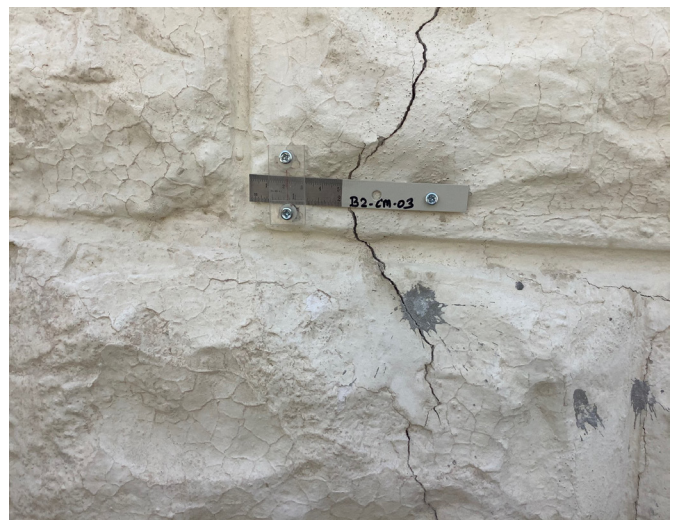
Model EDJ-40C Crack meter installed
